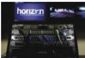
Video distribution is via HDBaseT interconnection, using an Atlona AT-UHD-PRO3-88M matrix as the control room hub
