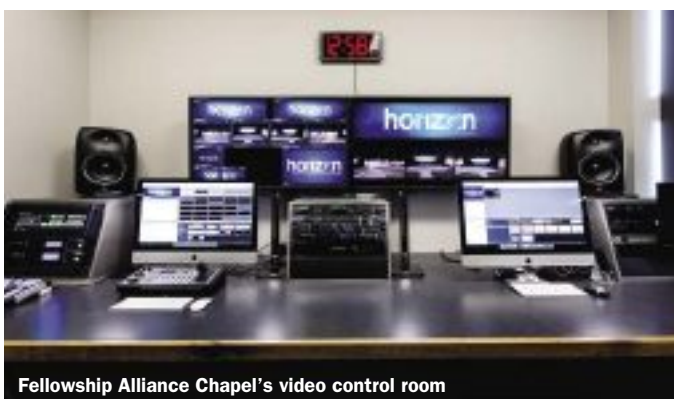
Fellowship Alliance Chapel's video control room
